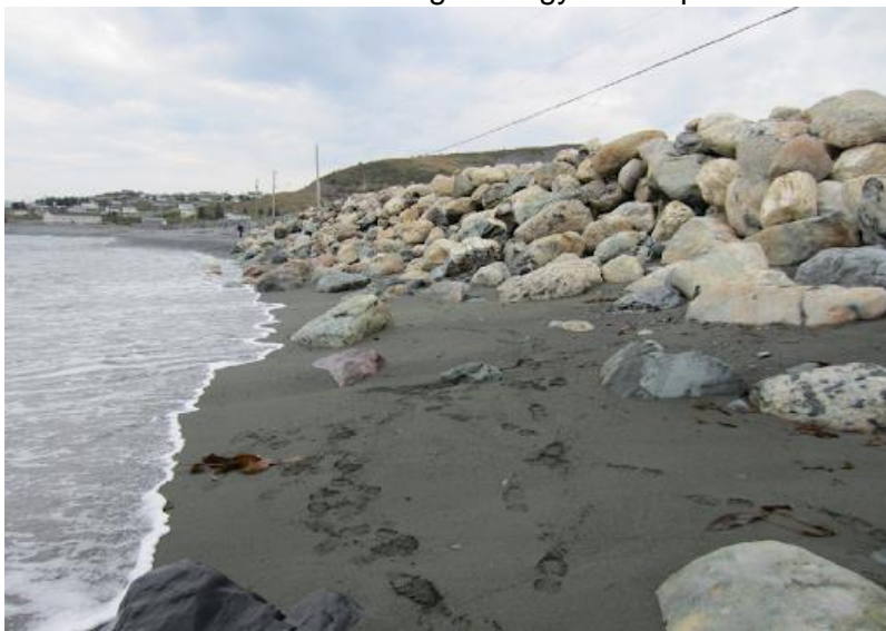
Figure 1.20 Riprap implemented in October 2011 along the west section of the Eastern Ferryland Beach, Newfoundland and Labrador (Catto 1 )
