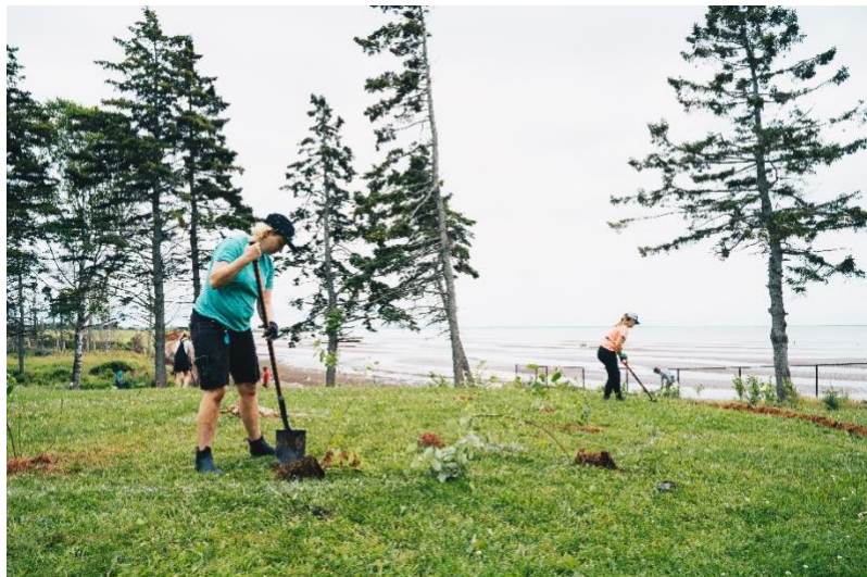
Figure 2.1 Members of PEI Watershed Alliance and partner organizations work on construction of living shoreline demonstration site (Stewart McLean)
