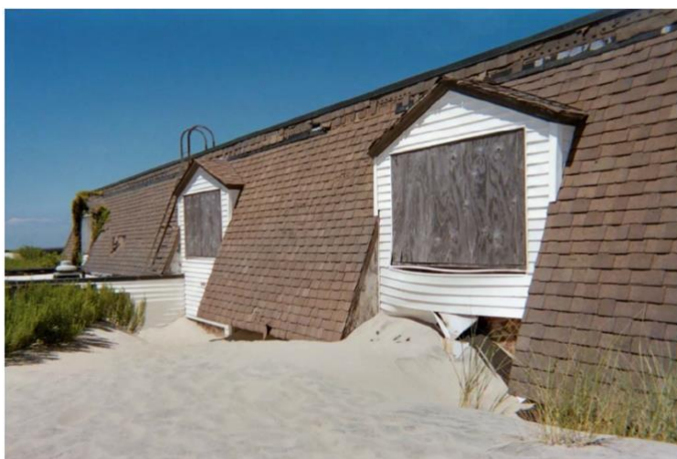
Figure 2.44 Abandoned coast guard station on Pea Island, North Carolina (Abandoned but Not Forgotten 265 )
