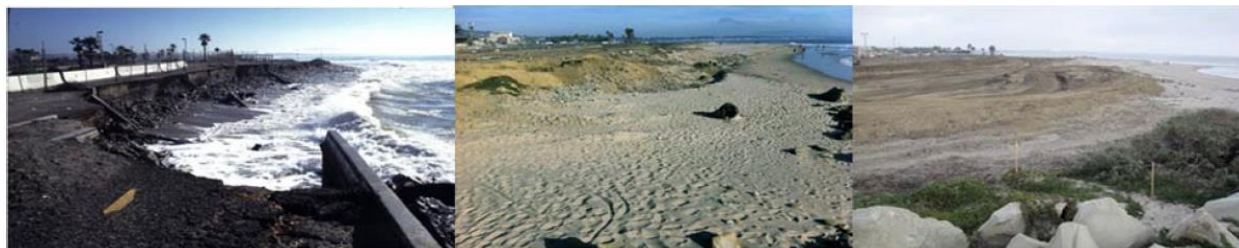
Figure 2.42 Managed retreat at Surfer's Point California. A damaged bike path and parking lot were removed to restore the Beach (P. Jenkin 260 )
