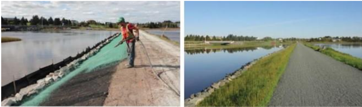
Figure 3.5 Installation of a turf reinforced mat with rock toe up to elevation of HW along coastal trail near Lawrencetown Beach, NS. It was infilled with hydraulically applied mulch (left), which was selected based on site conditions.
