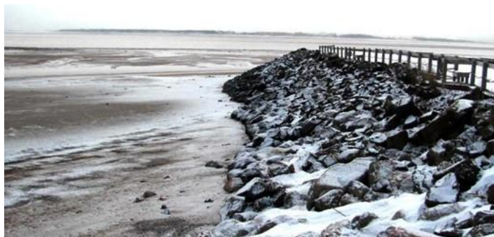
Figure 3.13 Rip-rap slope at Kingsport, NS, on the Bay of Fundy (Bruce Higgins, CBCL Limited)
