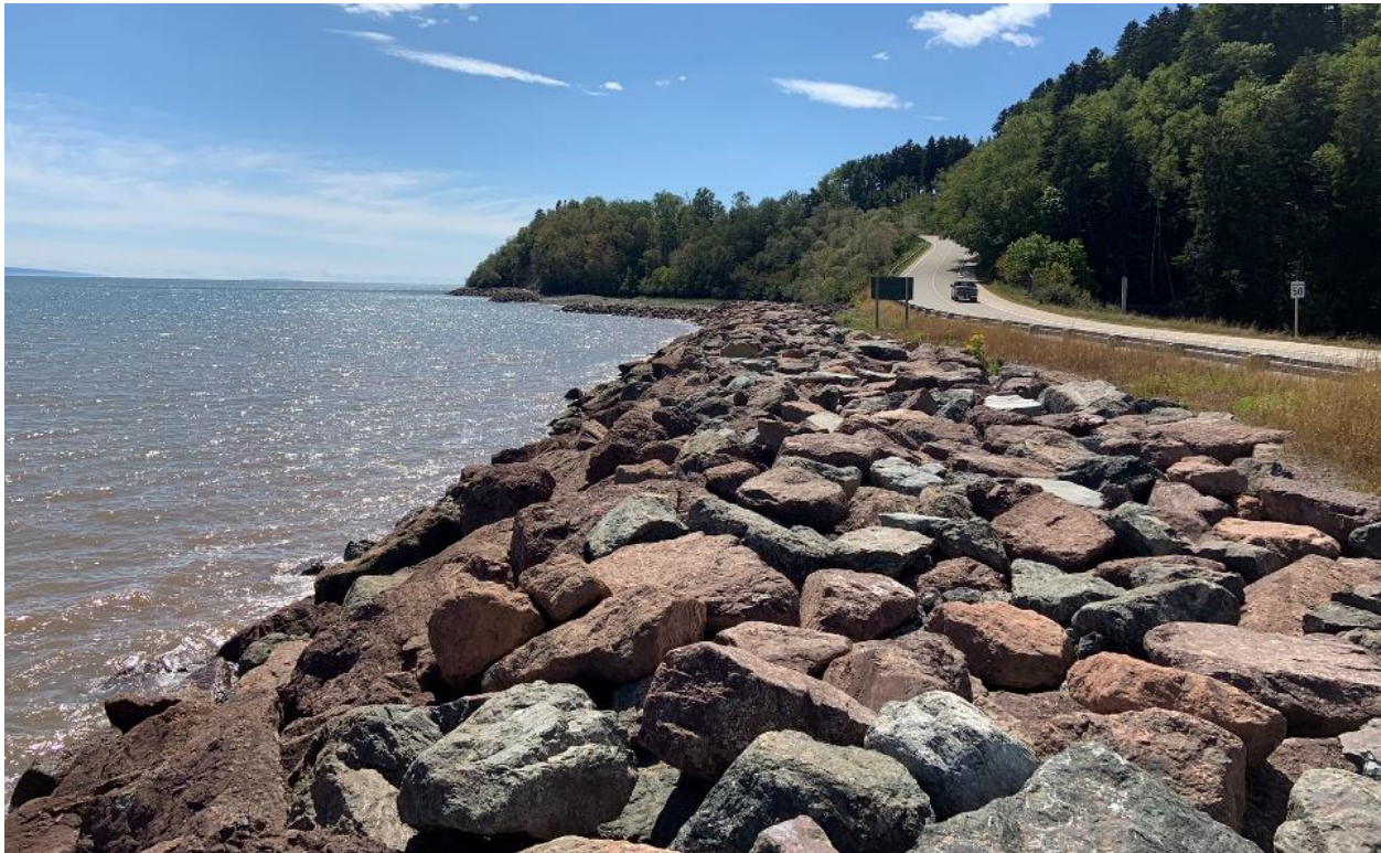
Figure 3.11 Revetment combined with beach stabilization structures at Fundy National Park, NB (Vincent Leys, CBCL Limited)
