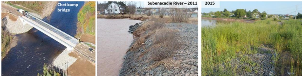
Figure 3.20 Scour protection at Cheticamp Bridge Piers using rock (left), and long tidal Shubenacadie River, NS (middle and right) using rock-filled gabion mats.
