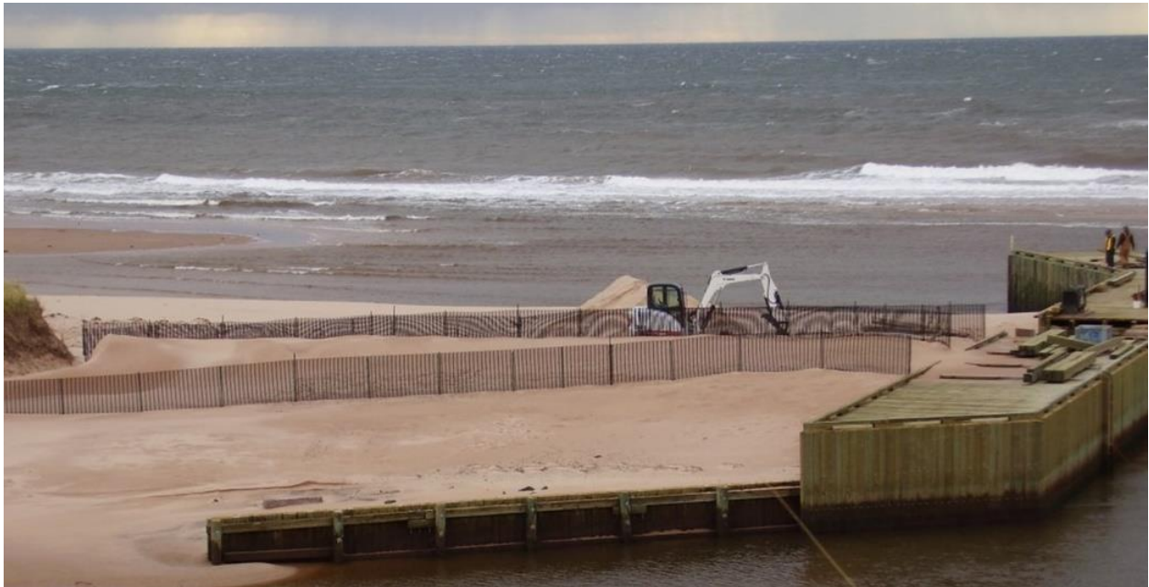
Figure 3.6 Dune restoration during the construction of a buried revetment at Basin Head, PEI (Jody MacLeod, CBCL Limited)
