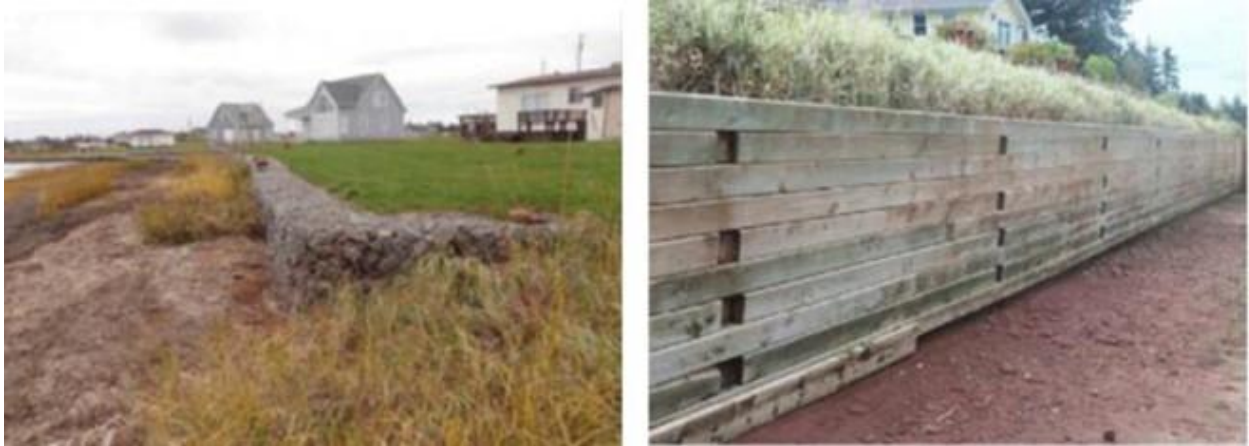
Figure 3.17 Retaining walls made of wire-mesh baskets or 'gabions' (left) and timber (right).
